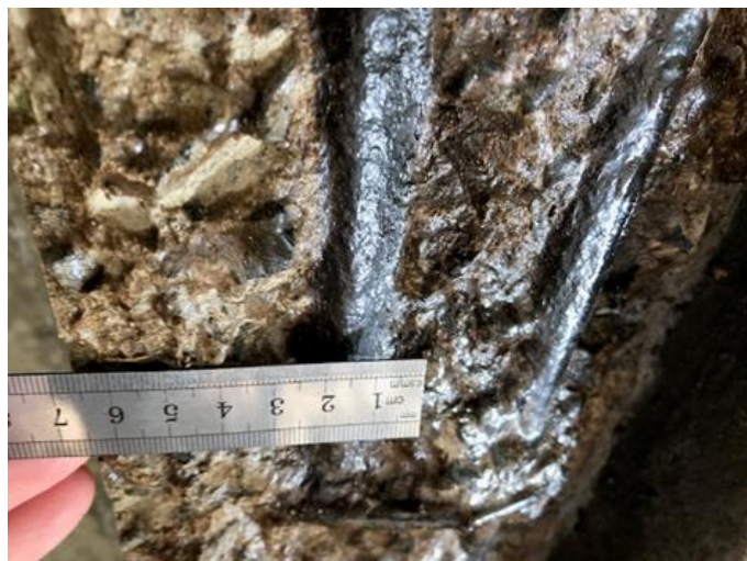
Image 1: Exposed reinforcing, spalled concrete section
